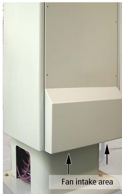
Fig. 27: Fans inlet. Remove snow, sedimentation,...
